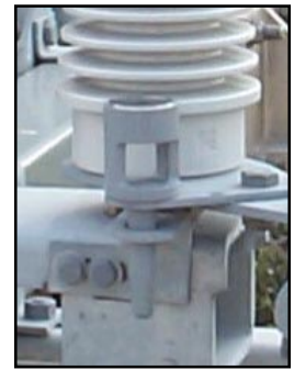
Switch Blocking Pin Installed in Switch
