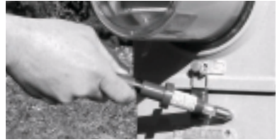
Testing a meter pedestal.
