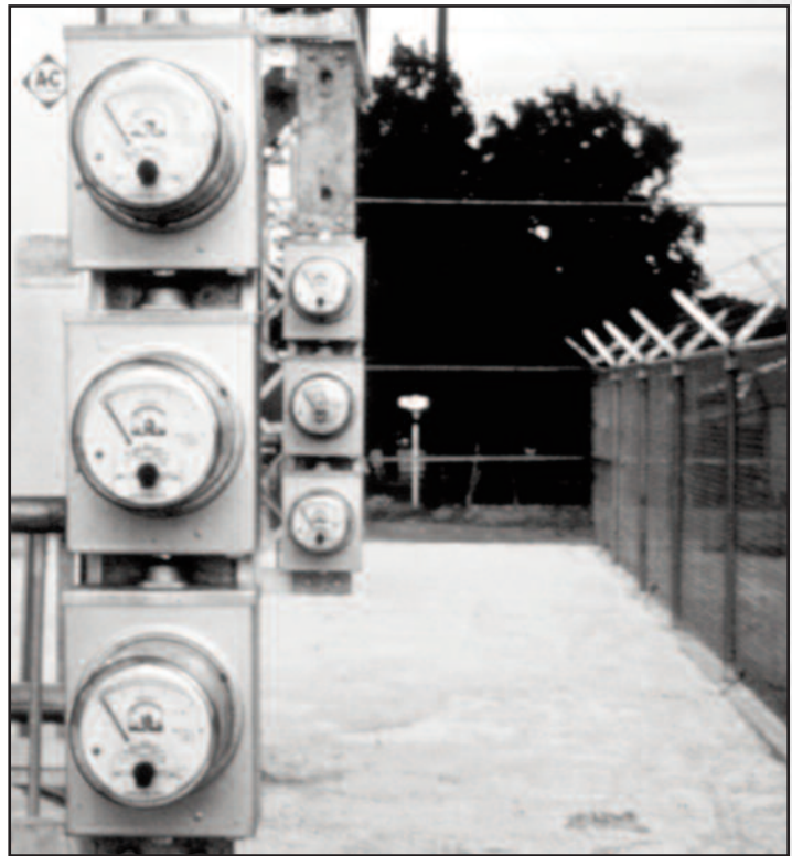
ADS-7 socket mounted version in substation application.
