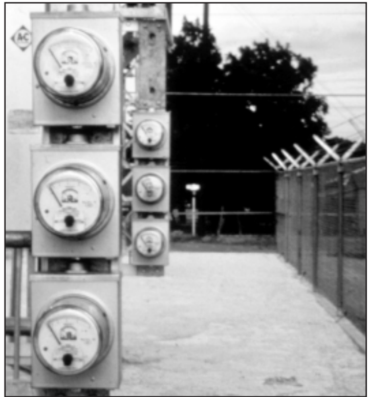
ADS-7 socket mounted version in substation application.
